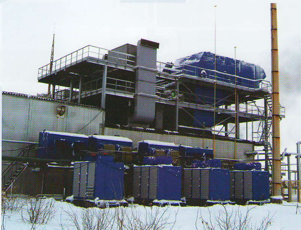
56 MW gas-turbine power plant in Zhanazhol, Kazakhstan
